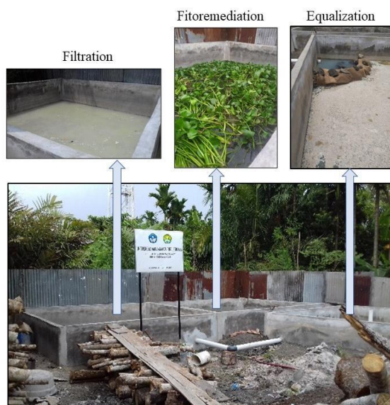
Fig 3. Application of tofu industrial wastewater treatment technology
